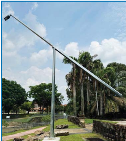
Mid-Hinge Pole Shah Alam, Selangor
