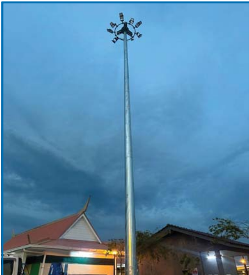
Highmast Pole Tanjung Sepat, Selangor
