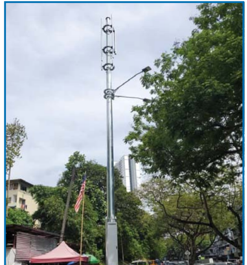
5G Monopole Kuchai Entrepreneurs Park, Kuala Lumpur
