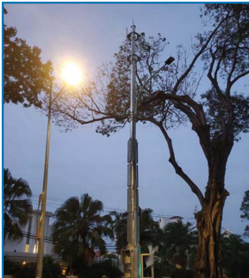
5G Monopole Jalan Kelawai, George Town, Pulau Pinang
