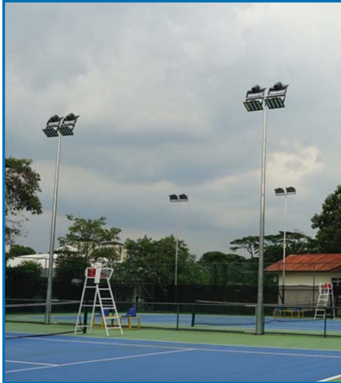
Floodlight Pole Tun Razak National Tennis Centre, Jalan Duta, Kuala Lumpur
