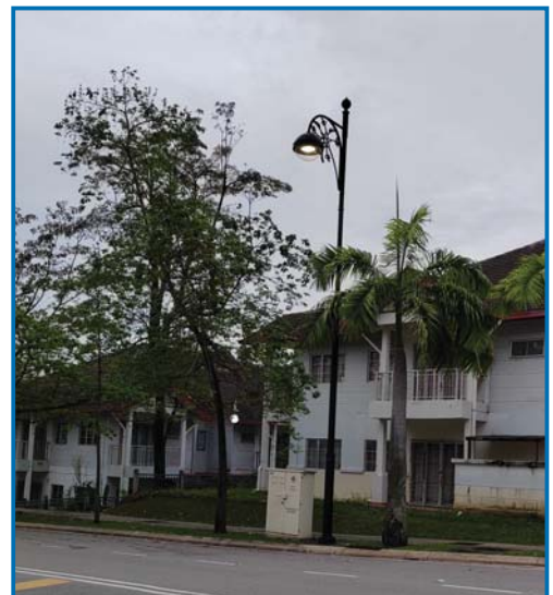
Decorative Pole Presint 11, Putrajaya
