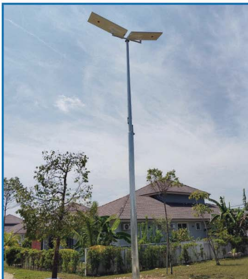
Solar Street Lighting Mid-Hinged Johor
