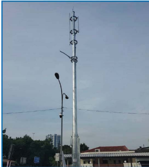
Smart Pole | Monopole Taman Kepong, Kuala Lumpur
