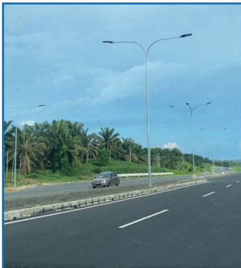
Octagonal Pole WP27 - Pan Borneo Highway, Sabah
