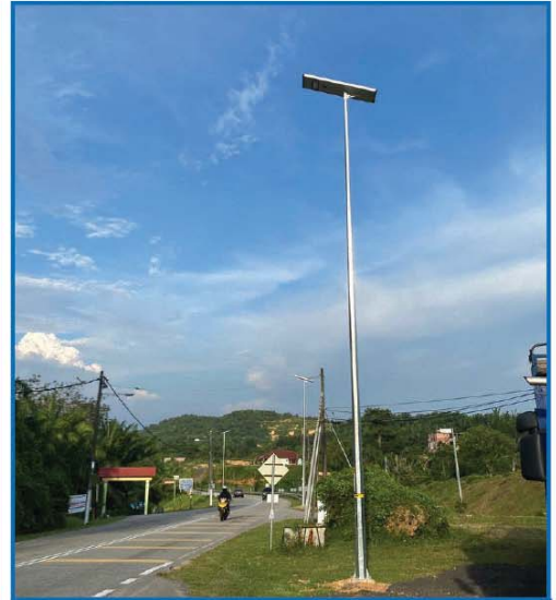
Solar Octagonal Pole Masjid Tanah, Melaka
