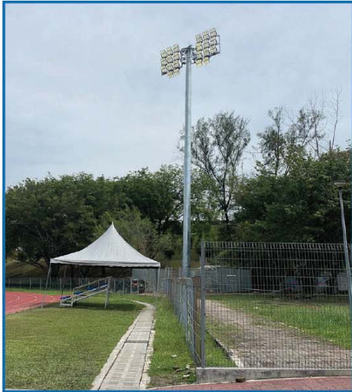
Highmast Pole Stadium Sultan Sulaiman, Klang, Selangor
