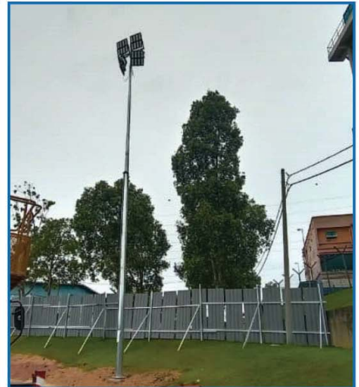
Floodlight Mid-Hinged Pole Stadium MPKJ, Bandar Baru Bangi, Selangor
