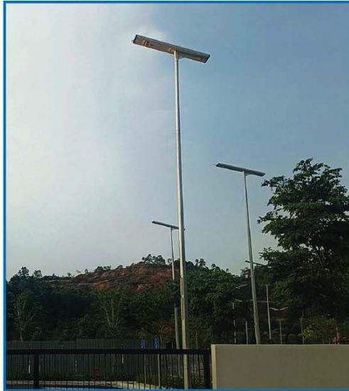
Solar Octagonal Pole Kota Emerald, Selangor
