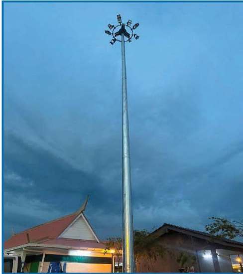
Highmast Pole Tanjung Sepat, Selangor
