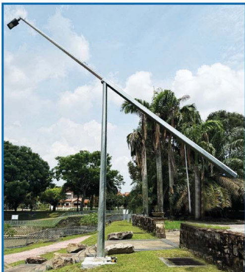
Street Lighting Mid-Hinged Shah Alam, Selangor
