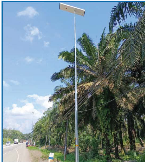
Solar Octagonal Pole Sg. Karas, Labis, Johor
