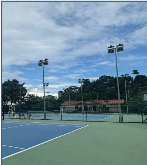
Floodlight Octagonal Pole Tennis Court, Kuala Lumpur
