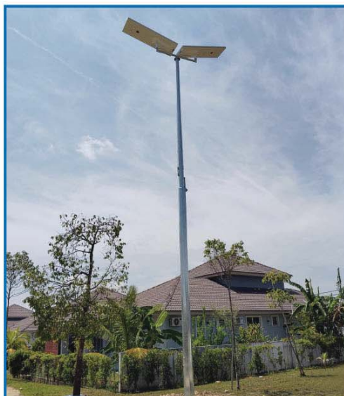
Solar Street Lighting Mid-Hinged Johor
