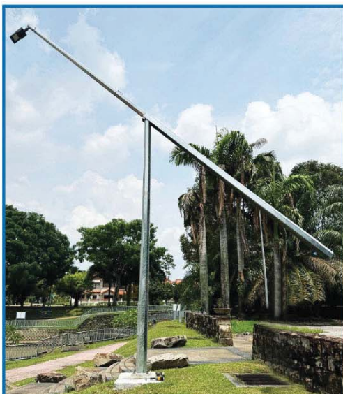
Street Lighting Mid-Hinged Shah Alam, Selangor
