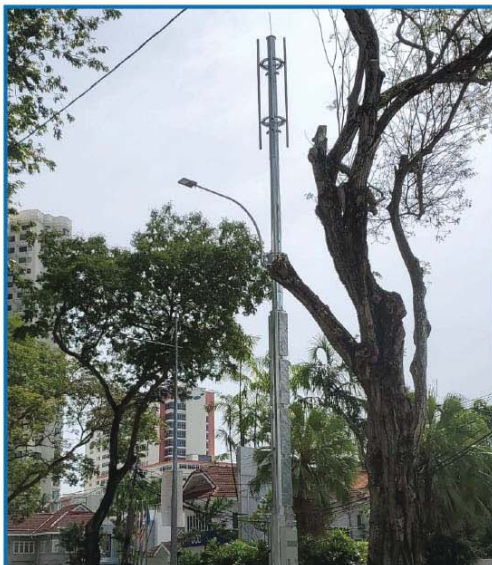
Smart Pole | Monopole Persiaran Gurney, Pulau Pinang
