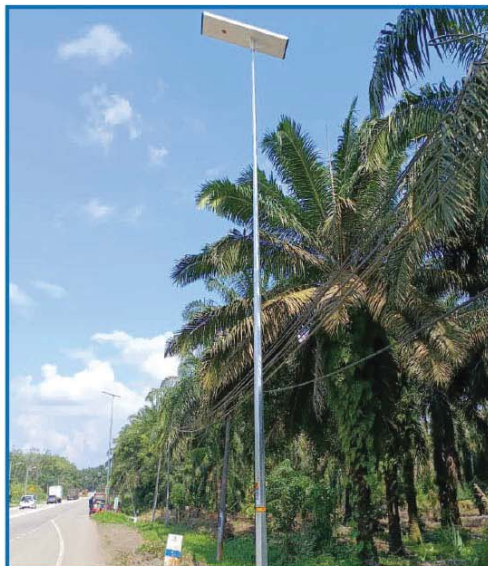
Solar Octagonal Pole Sg. Karas, Labis, Johor
